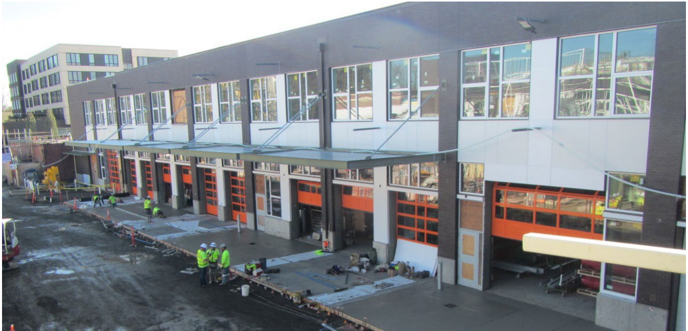
Above: View southeast, exterior of Building H auto shops. Note the concrete driveway aprons were being placed this day. The auto shop doors are orange with glass panes. (Photo courtesy of Gerry Ochs.)
