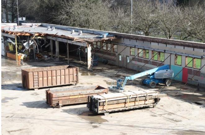
Above: Bound trailer loads of timber salvaged from demolition for Benson Tech modernization. They will be recycled for other uses.
