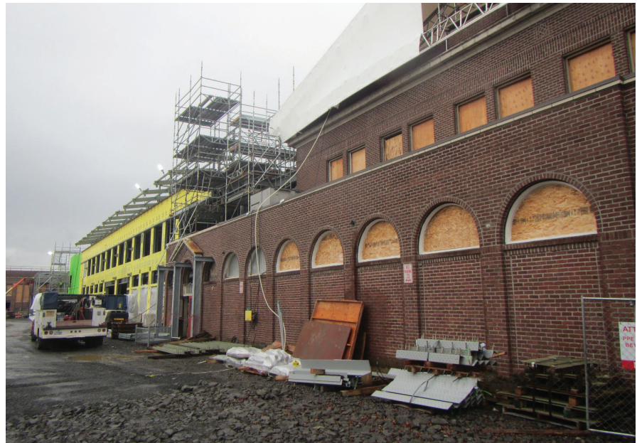
Above: The seismic upgrades of shotcrete shear walls, around the inside perimeter, are in progress in Foundry Building D. (Photos courtesy of Gerry Ochs.)
