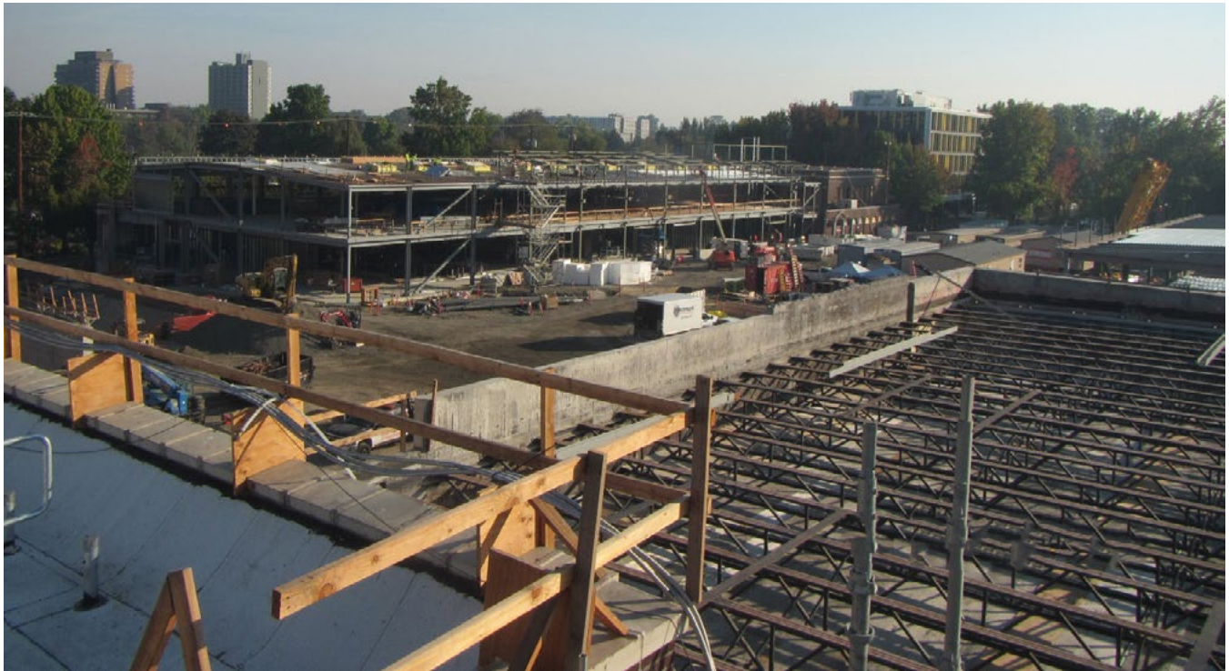
Above: Overall view NE. Building C is in the background. In the foreground to the right is the roof truss system over the Main Gym. The Main Gym roof replacement is ongoing.
