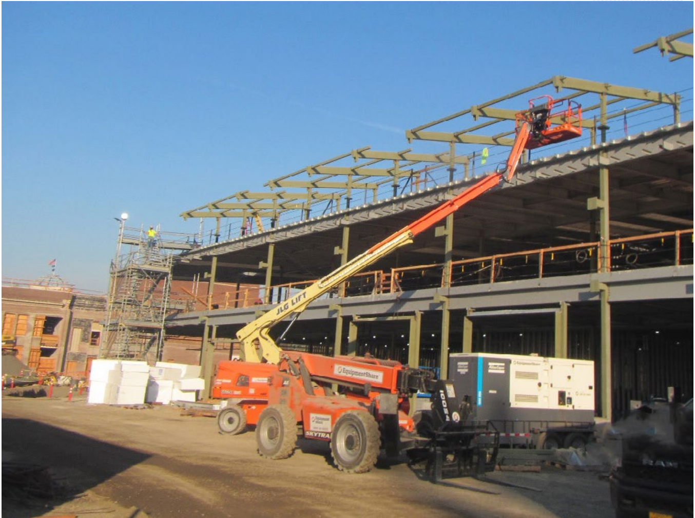
Above: View NW of the progress on Building C. Approximately 98% of the steel framing components are now in place. Solar panel brackets are visible along the roof edge. Solar panels will also be installed on portions of this south-facing exterior wall.
